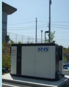
Kobe renewable energy hydrogen station
